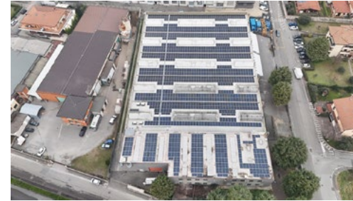
Daikin Compounding Italy introduced solar power generation system at its factory
